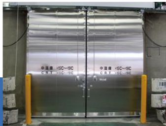
Mid-range Temperature room (+15°C ~+19°C) : 161㎡
