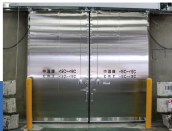
Mid-range Temperature room (+15°C ~+19°C) : 161㎡
