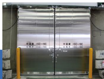
Mid-range Temperature room (+15°C ~+19°C) : 161㎡
